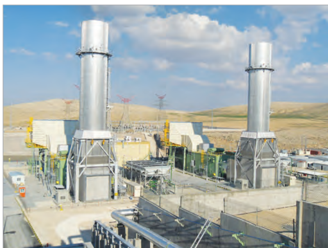
Samra Gas Turbine 140MW×2units Power Plant (Jordan)
