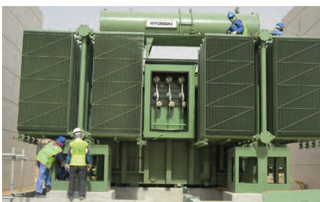
Step-Up TR, 11/230KV 40 MVA
