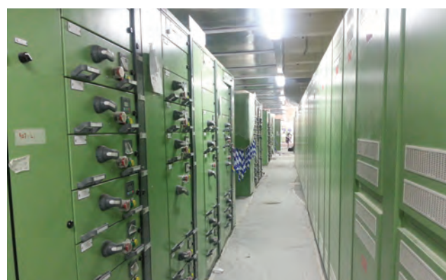
Sub Station LV SWGR/MCC Room
