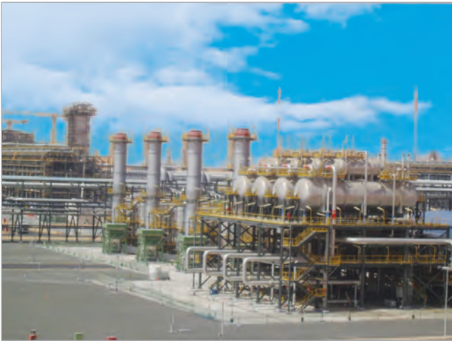
Shah GAS U&O Project - Instrument (UAE)
