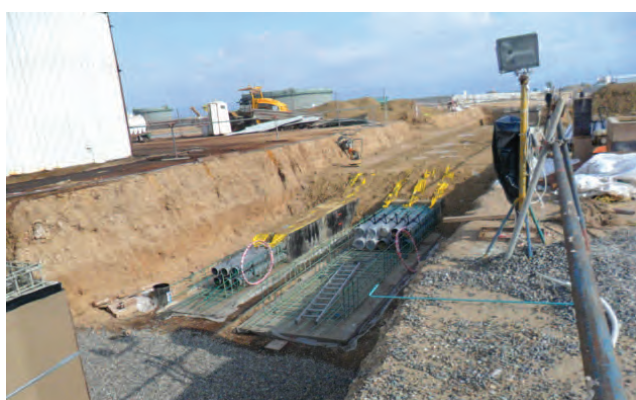
Duct Bank for HV Cable
