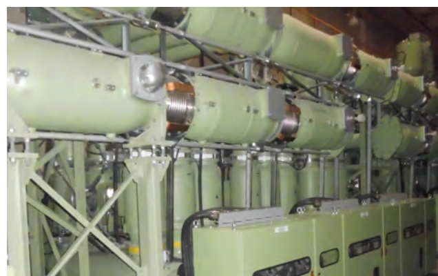
220KV GAS INSUL. BUS DUCT
