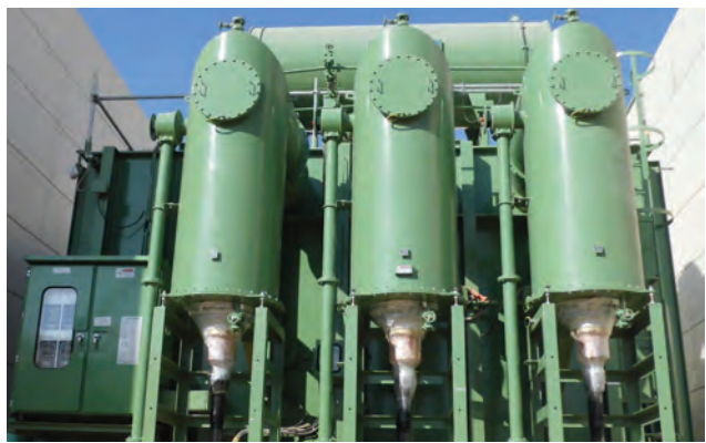
Auxiliary Transformer 13.8/6.9KV 20/25 MVA
