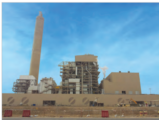
Marafiq STG Units 250MW×2units Power Plant (KSA)
