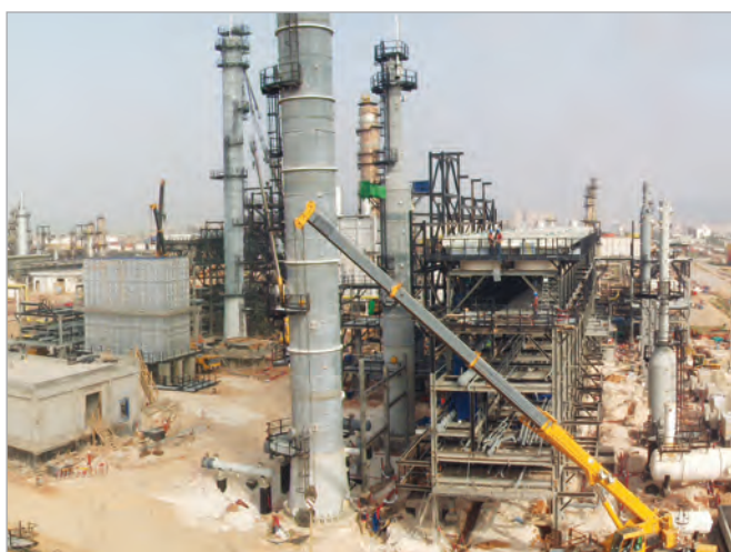
Arzew Refinery Project ( Algeria )
