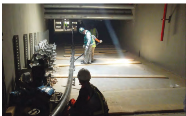
33KV Power Cable 1C-630sqmm
