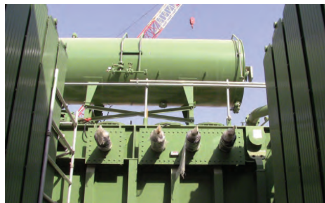
Step-Down TR, 220/33KV TR. 100/133MVA
