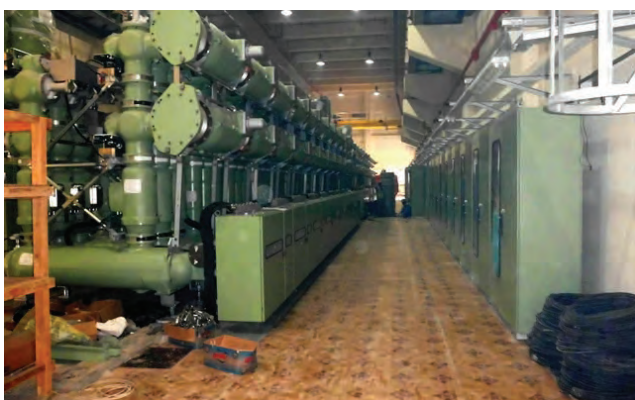
GAS Insulated Switchgear Incoming Feeder 2,500A
