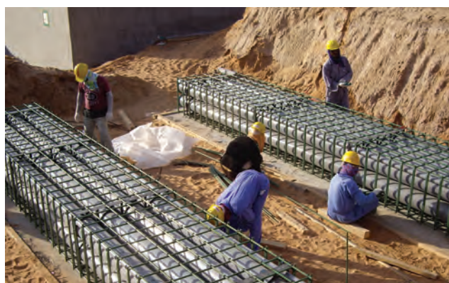
Duct Bank for HV Cable
