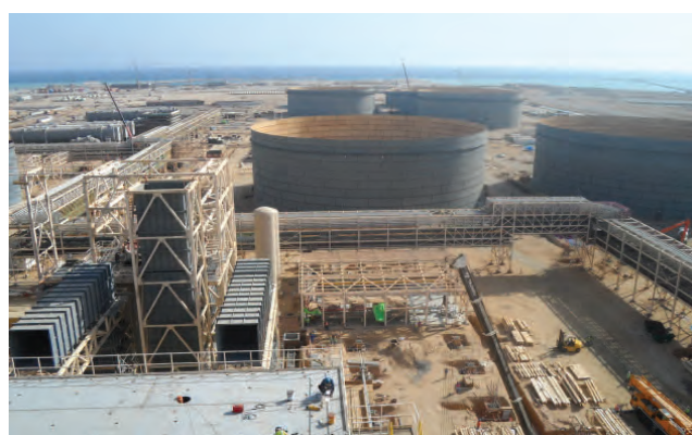
Pipe Rack For Cable Tray
